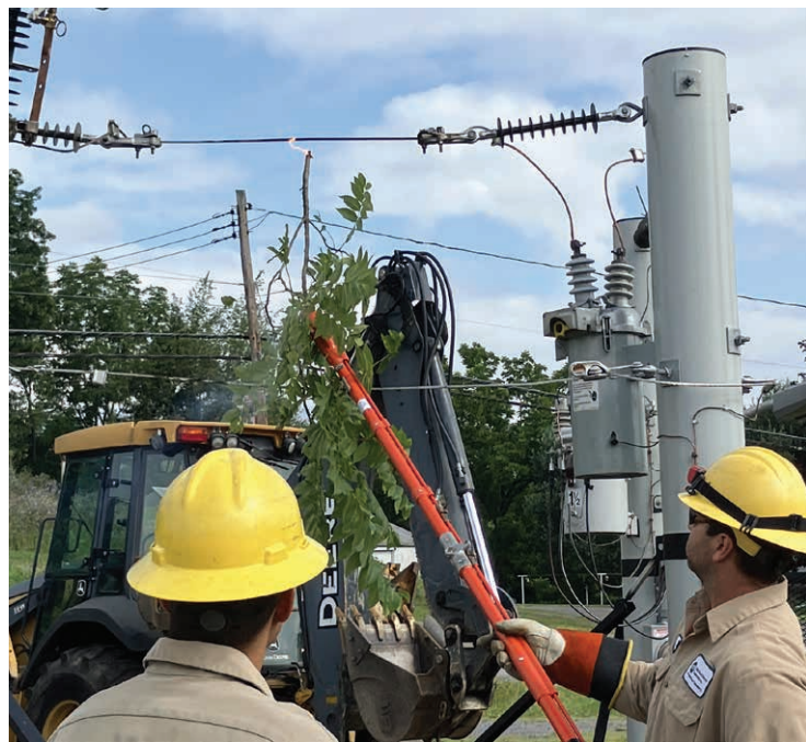
ALL CLEAR?: Valley Rural Electric Cooperative Linemen Matt Fish, right, and Riley Price use a tree limb to draw an arc during a safety presentation. The cylindrical device above Matt's right hand is an automatic recloser, a piece of equipment that prevents a short-duration or transient fault from causing a power outage.
