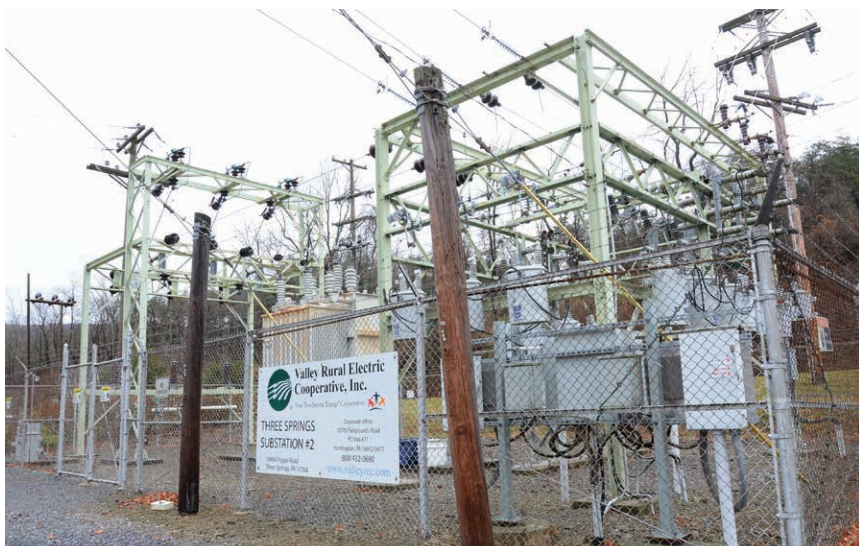
ABOVE: Valley REC will replace the aging Three Springs substation this year with a new facility in the same location in Cromwell Township, Huntingdon County.
